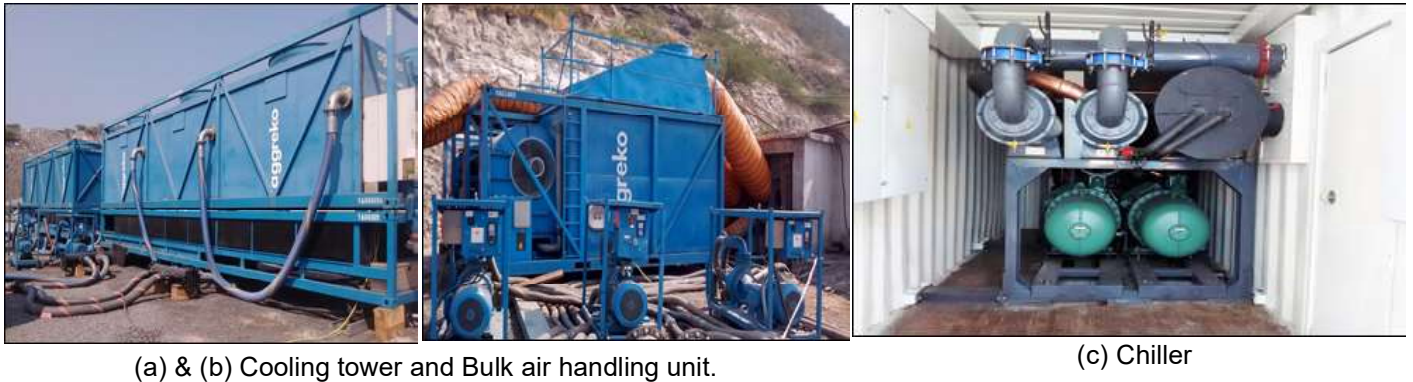
Fig.3: The overview of Bulk air handling cooling system equipment
